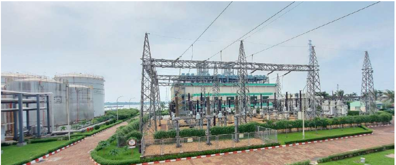
Midland East Power Limited - 150 MW (net) HFO based power plant at Ashugonj, Brahmanbaria.
